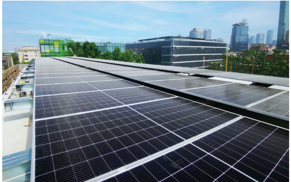
Taikoo Li Sanlitun in Beijing is the first commercial building in the Chinese Mainland to install a Photovoltaic, Energy Storage, Direct Current, Flexible ("PEDF") system. This image shows solar panels positioned on the mall's roof.
