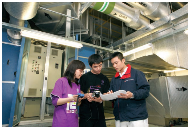
Tsinghua University students have the opportunity to gain hands-on engineering experience, working alongside Swire Properties’ maintenance teams.
